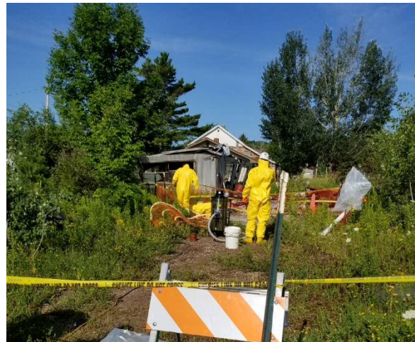
EPA crew cleaning up mercury spill at abandoned repair facility garage in Mass City (Source: WLUC/Ontonagon County Emergency Management Coordinator)
