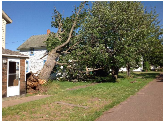
Storm damage from thunderstorm wind on July 21, 2016 in the Village of Ontonagon (Source: NWS Marquette).
