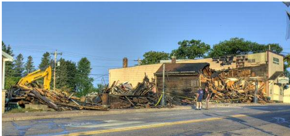
Damages due to the 2008 Labor Day fire in the Village of Ontonagon (Source: Henry Kisor )
