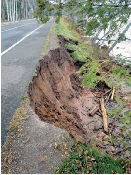
CR107 washout near the Porcupine Mountains Wilderness State Park (Source: Michigan DNR)
