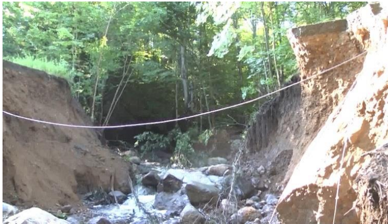
Stagecoach Road washout due to beaver dam collapse on July 18, 2017 in Baraga County. (Source: ABC 10 News)
