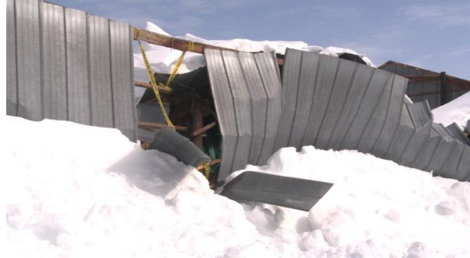
Baraga County fairground roof partially collapsed due to heavy snowfall in March 2019 (Source: Megan O'Connor, Upper Michigan Source)
