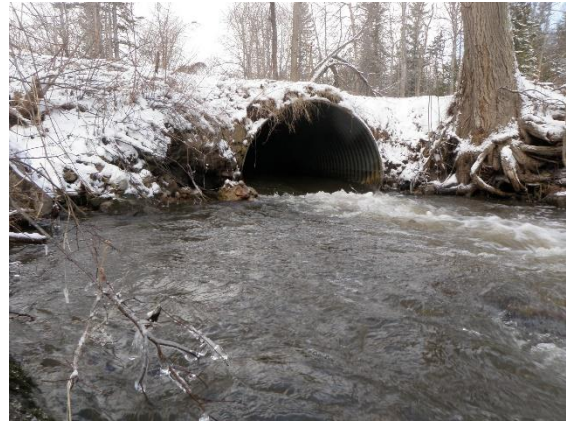
Upgraded culverts can mitigate flooding problems by increasing the flow capacity of streams as they pass under roadways.
