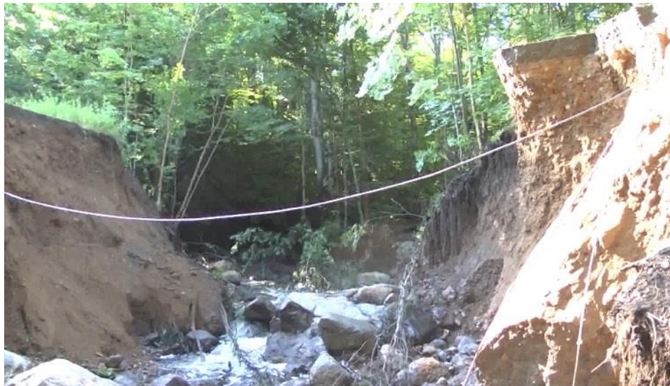
A Beaver dam collapse caused major road damage on July 18, 2017 (Source: ABC 10 News)
